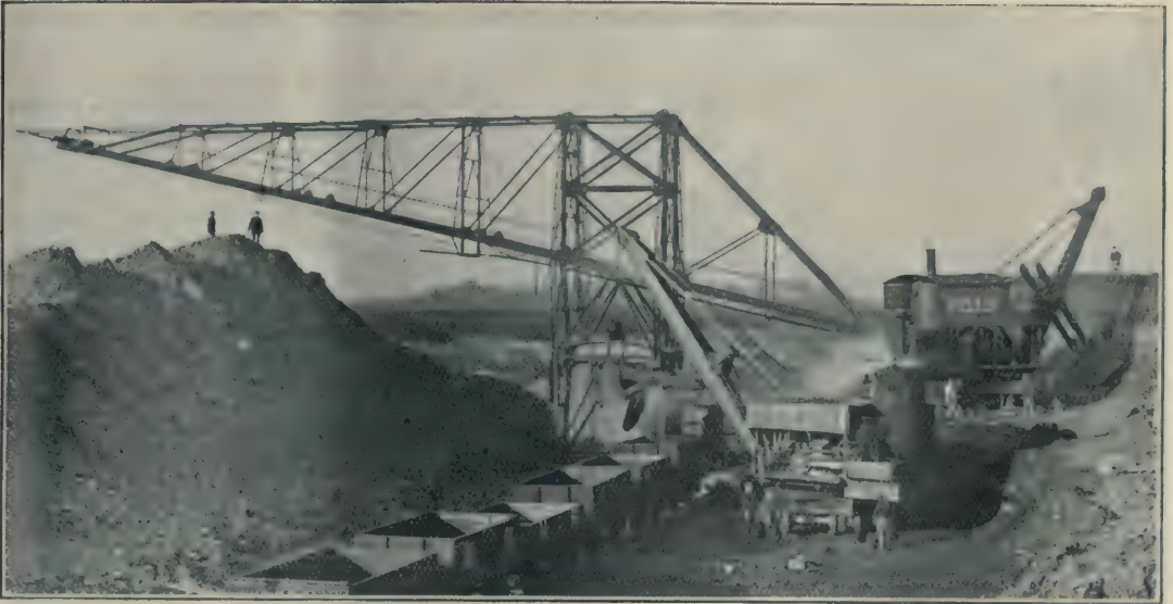
FIG. 2—The upper machine at the right-hand corner is excavating the cover; the material is sent by the transporter across to the other side of the cutting; the lower machine at the right-hand side is excavating the iron ore and leading it into the wagons.
